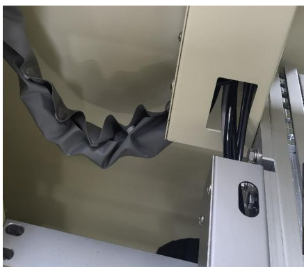
Protection for all connecting wire
